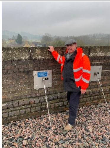
Our President , on a cold day, inspecting the plaque, attached to the restraining plate preventing the parapet from moving any further
