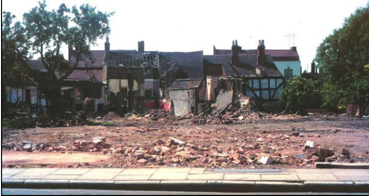
Figure 61: 89 to 83 High St. (LtoR), seen from the Oldbury during demolition in 1965. (Bigland)
